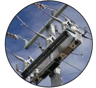
Automated Feeder Switches
